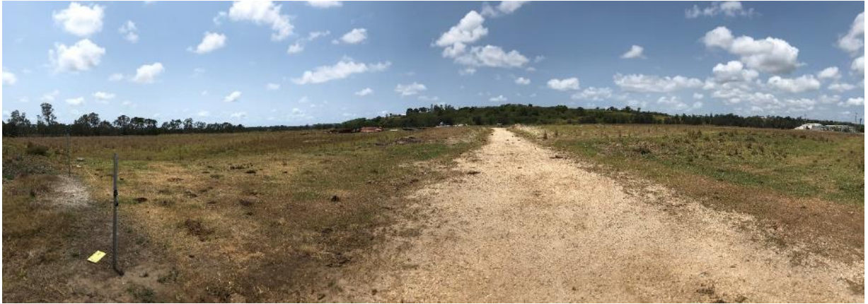
Photo 6. Haul road were stabilised and no signs of dust generation during site inspection.
